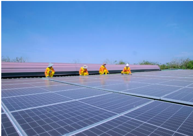
SOLAR ROOF TOP POWER PLANT
